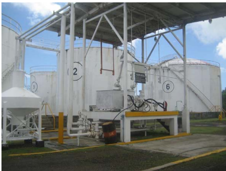
Figure 7-1. FSM Petroleum Corporation Fuel Facilities
