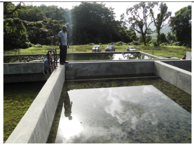
Treatment Plant for Utwe Water System
