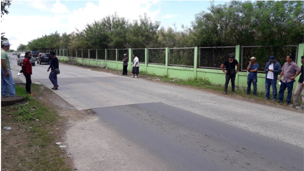
Inspecting Defects in the Weno Road during Pre-Bid Meeting With Contractors
