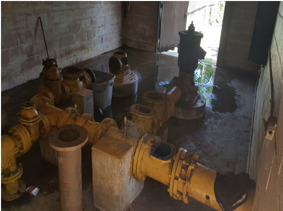
Pump House dysfunctional Jan 2018
