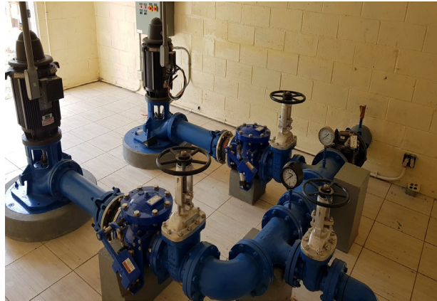
Pump House with new pumps, pipes and valves
