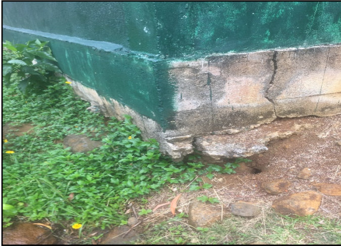
BLDG 1: FOUNDATION FLEXURAL CRACK
