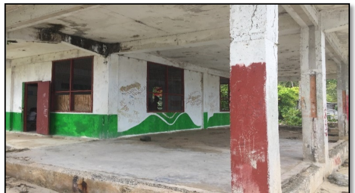
BLDG 1: MAJOR CRACK AT COLUMN 1
