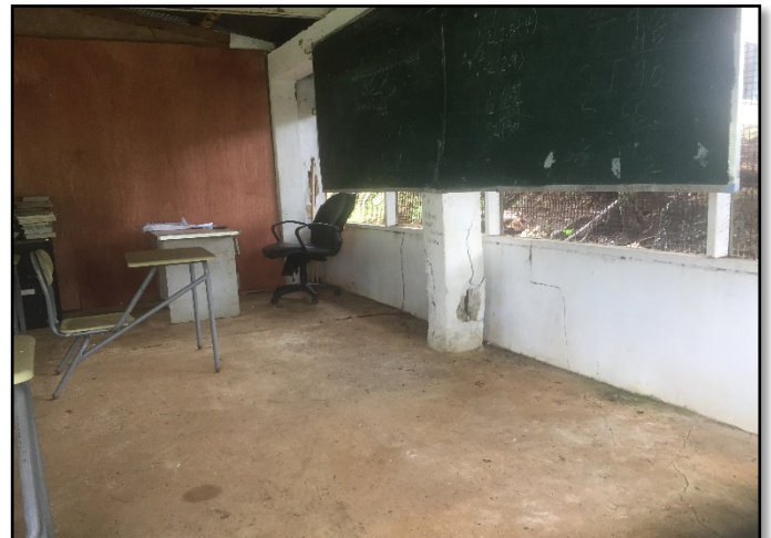
BLDG 1: MAJOR CRACK AT COLUMN 2
