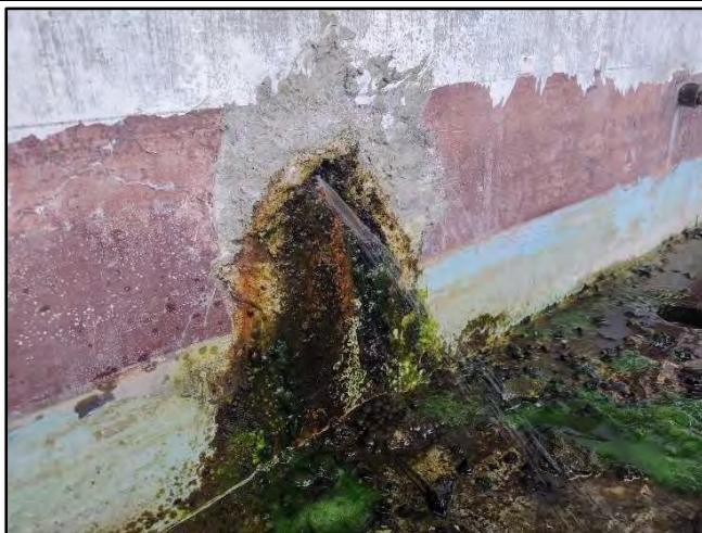
WATER LEAKING AT TOILET AREA
