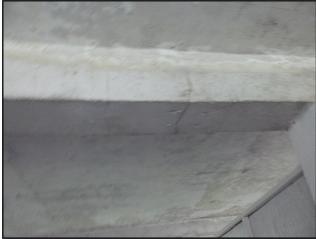
TENSION CRACK ON BEAM AT BLDG 1
