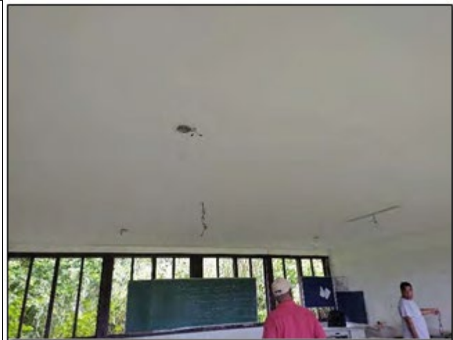
NO CEILING FANS AND LIGHTS
