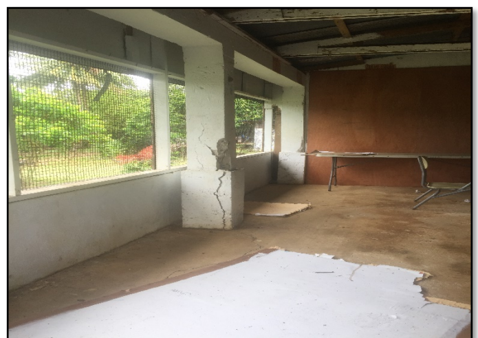
BLDG 1: MAJOR CRACK AT COLUMN 1
