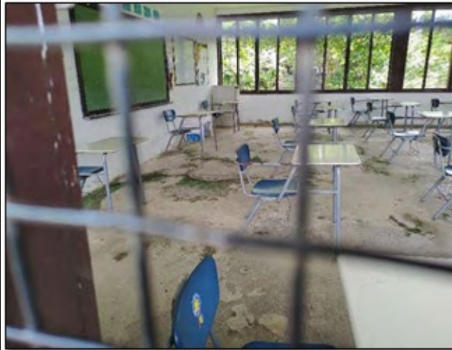
ALGAL GROWTH INSIDE CLASSROOM DUE TO FLOODING
