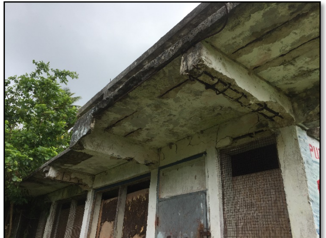
CONCRETE SPALLING AT BLDG 2
